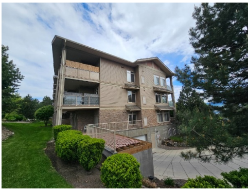
Before Picture showing the Left Side (West Side) of Building 3 Showing Wood Trim to be Painted
