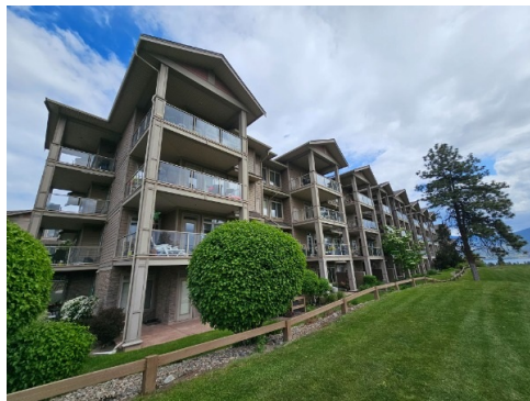
Before Picture showing the Rear Side (West Side) of Building 1 & 2 Showing Wood Trim to be Painted
