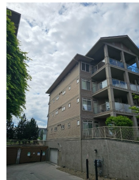
Before Picture showing the Left Side (South Side) of Building 2 Showing Wood Trim to be Painted
